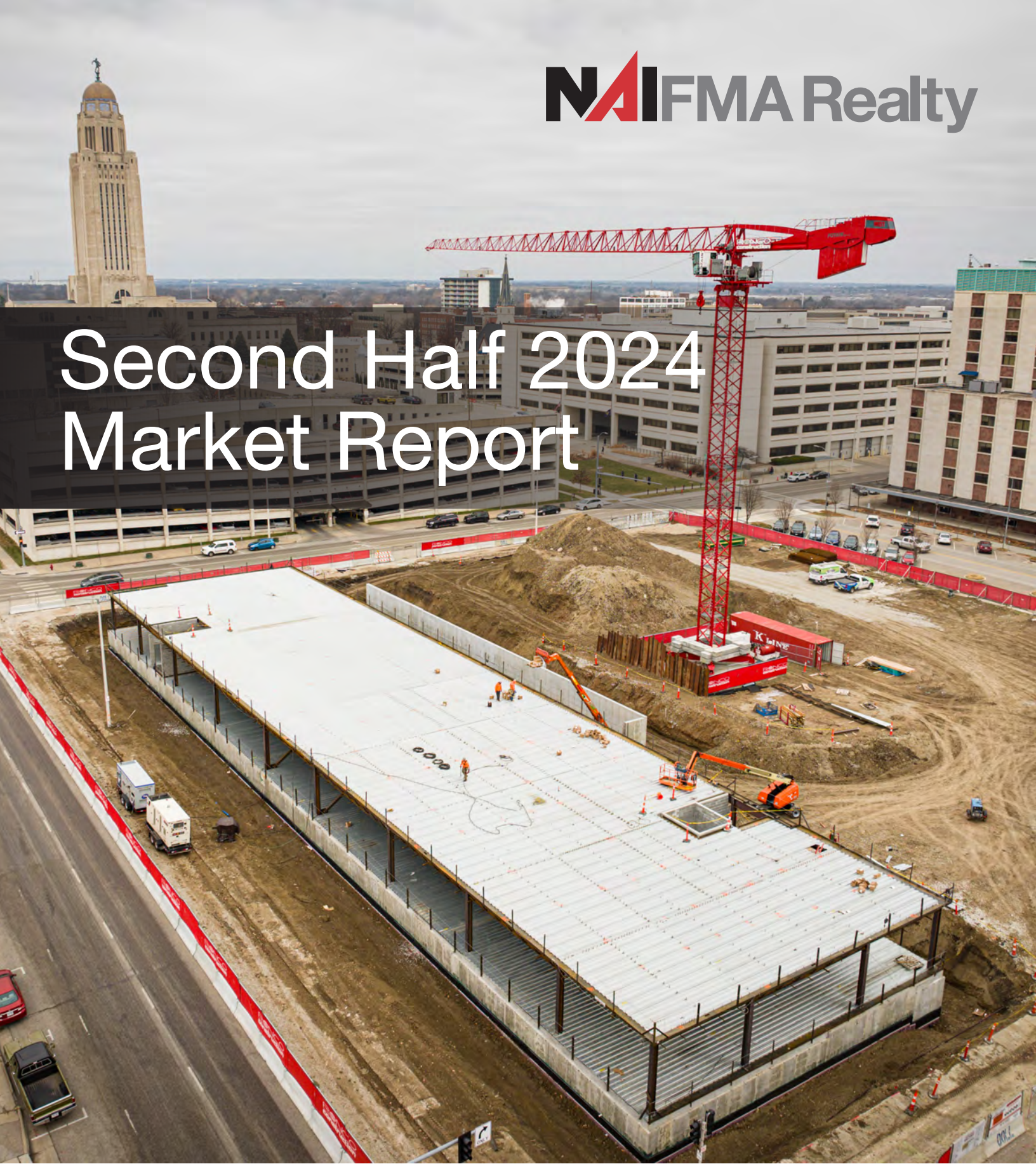
Image: MURAL, a mixed-use development project under construction by White Lotus Group (Photo Courtesy of RONCO Construction)
